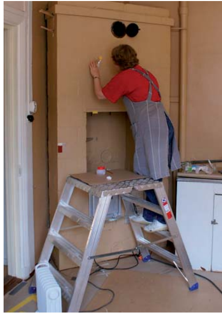
Conservator Raiili Laakso (above) working on the interior of the Worker Housing Museum (below), currently closed for refurbishment.
