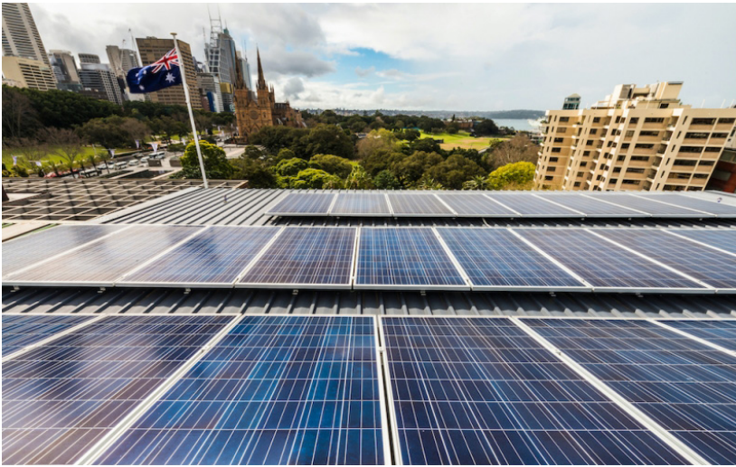
Solar panels on the roof of the Australian Museum. © Abram Powell/ Australian Museum
