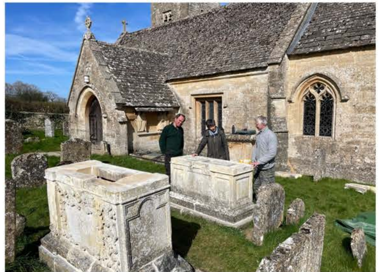
FIGURE 3. Churchyard of St Peter's, Little Barrington. Graham O'Hare (right) discussing the progress of works with Jacky King and Jan De Haldevang. Image: Adam Klups
