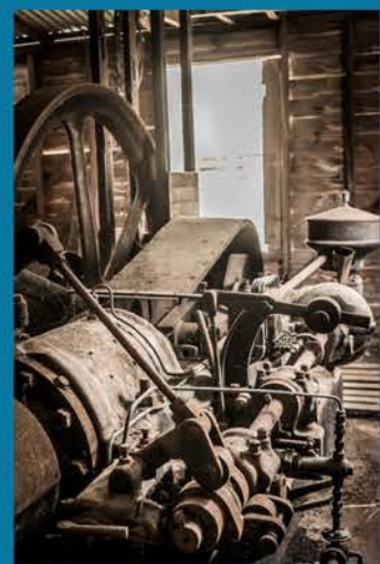
Original machinery inside the engine room 2018 / photo Naomi Creek
