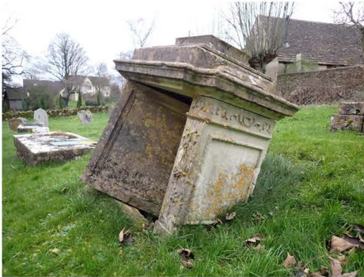
FIGURE 2. Churchyard of St Bartholomew, Nympsfield. A 'tea caddy' style tomb in the state of near collapse. Image: Graham O'Hare
