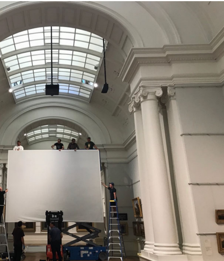
10-metre-high projection screen being suspended from the roof in Art Gallery of New South Wales 19 th century “old court” 2020. Image by Asti Sherring.
