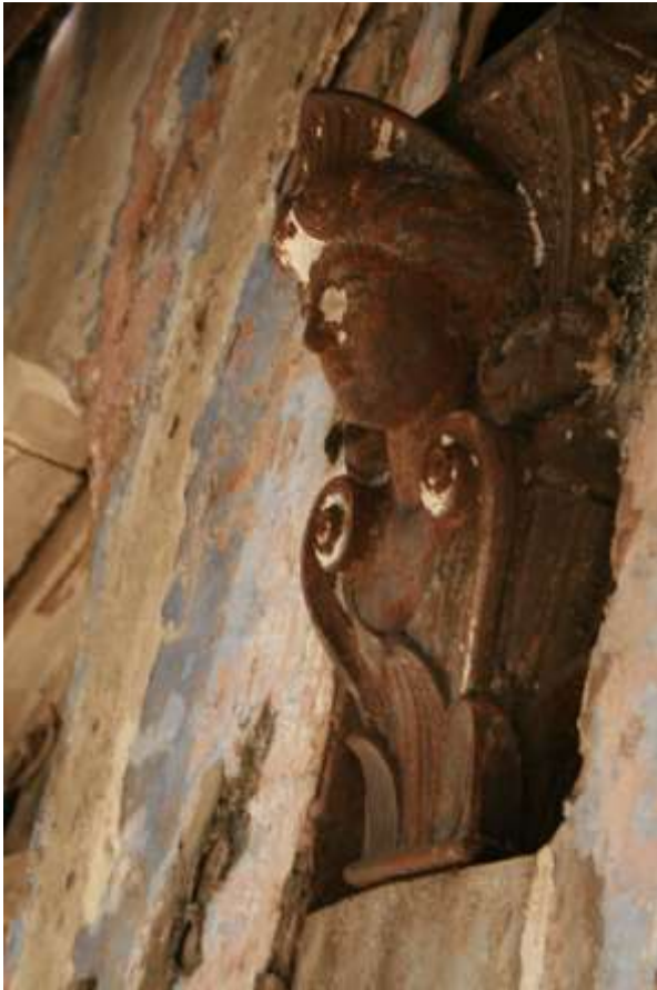
An example of the remaining decorative cast iron
