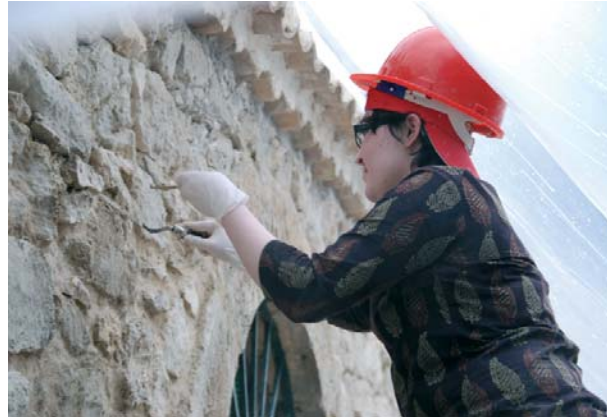
Not even the rain can stop us from saving the stone masonry!
