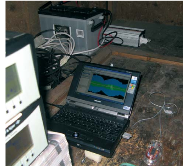
Monitoring set up
