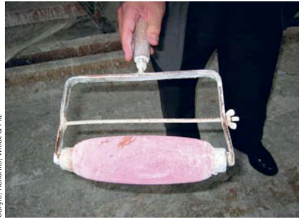
Claessens distinct orange peel texture is achieved using a specially made velvet-plush roller for the final layer
