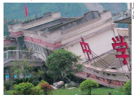
A school in Yingxiu town, Sichuan province after the earthquake.
